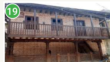
19. Sata Falcha: The public rest house reconstructed by Praya Sampada Project offers space of various public activities for the Sata neighbourhood.
